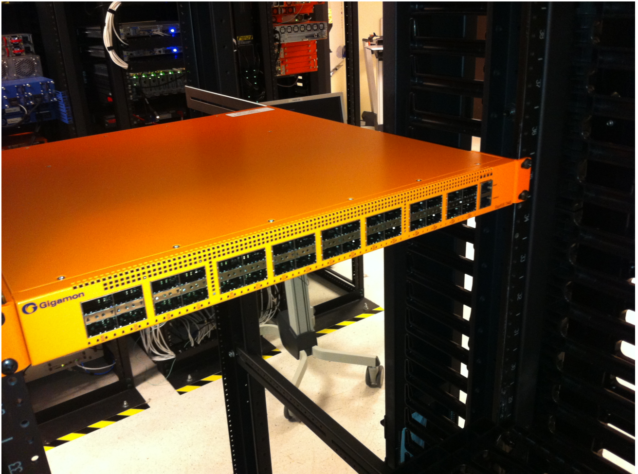
Figure 3 Front View of the Mounted Node to the Four-Post Rack
